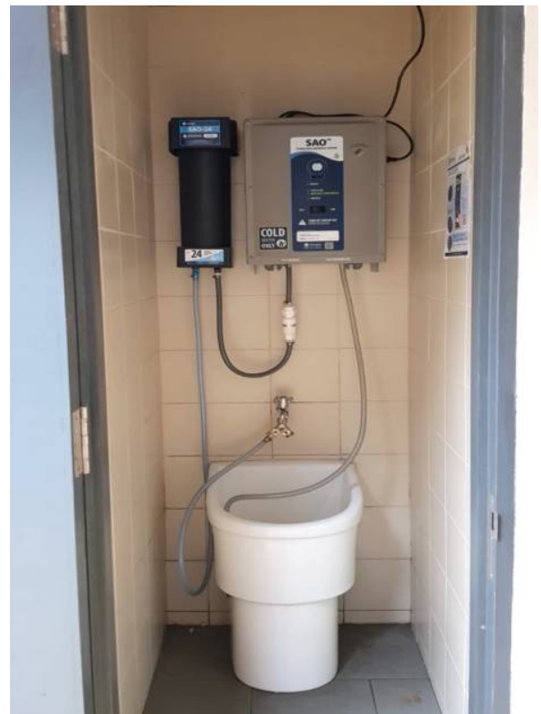
Tersano LotusPro installed in a janitor's closet
